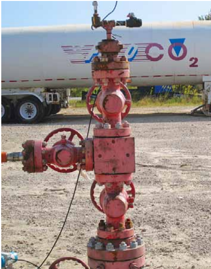
An injection well marks the site of a carbon sequestration research project at Mississippi Power's Plant Daniel, where 3,000 metric tons of CO 2 were injected into a deep saline rock formation below ground.
