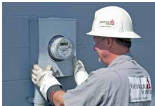
More than 3 million smart meters have been installed across the Southern Company system.
