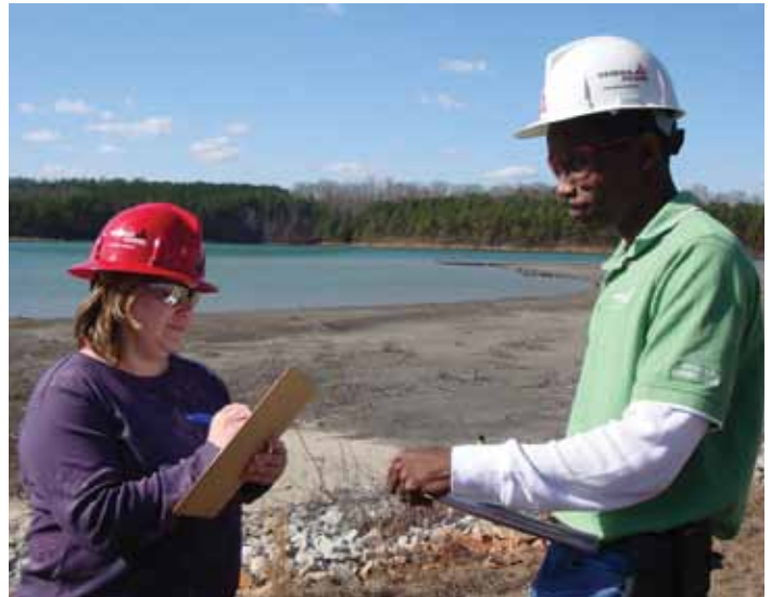
Compliance specialists Christy Garrett and Ron Goldsby inspect a dam, part of the regimen to ensure safety.
